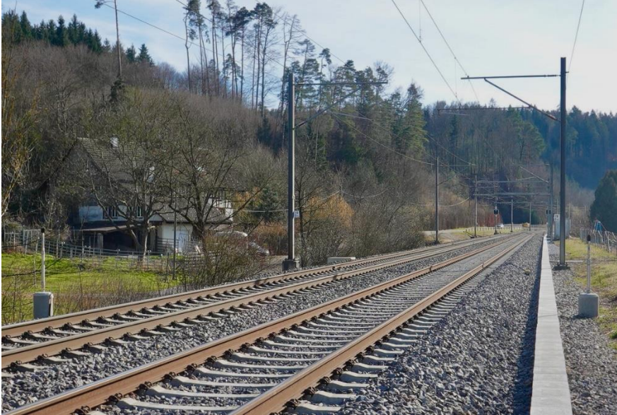
Figure 1: Photo of a noise monitoring station on the line between the cities of Zürich and Winterthur in Switzerland. The microphones can be seen on the left and right edges of the image. Data acquisition is performed in the gray box in the background, partially covered by the catenary mast on the right side of the track. Photo credit: own work by the author.
