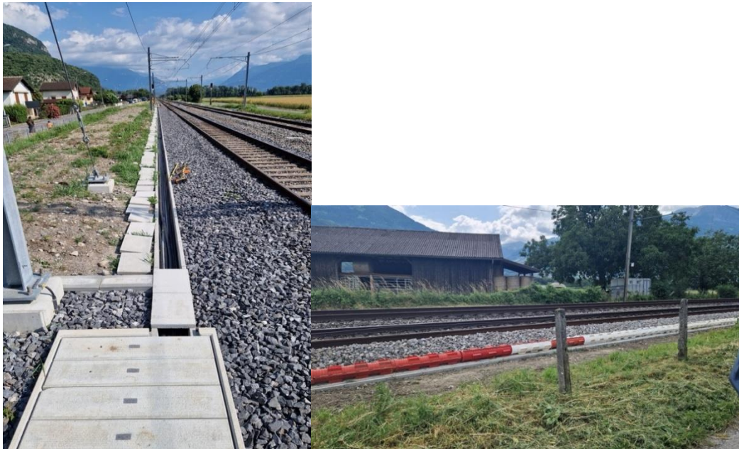
Figure 4: Examples of fiber conditions along the monitored railway corridor. Most sections (left) consist of buried telecommunications cables installed alongside other utilities, whereas some locations (right) showed cables positioned at the surface within temporary ducts. These differences may influence local coupling conditions and recorded signal amplitudes.
